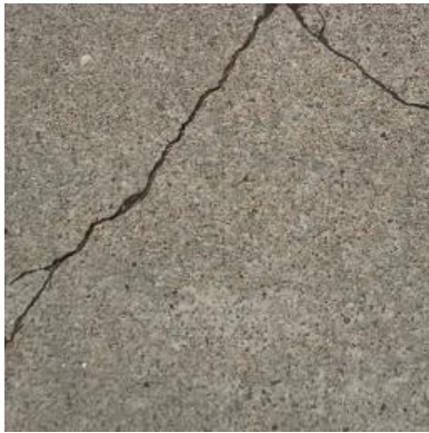
Figure 38 - g(x,y) image of cracked Concrete
